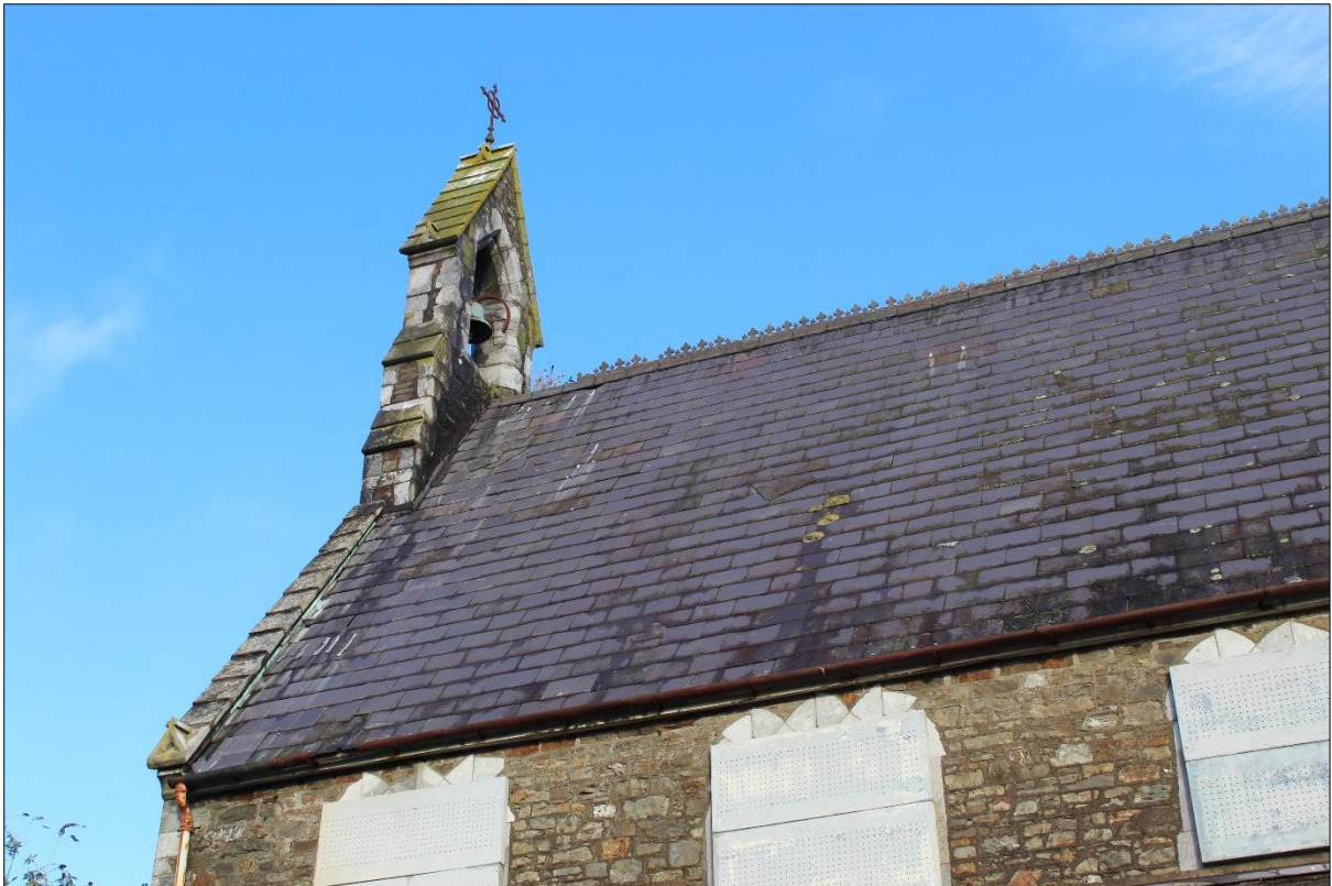
Plate 3: Detail of western bell-cote, localised loose slates and cement-pointed, weathered masonry of southern clerstorey.
