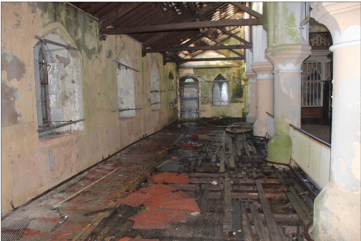
Plate 22: View to west along southern aisle with decayed timber floor that formerly held pews and geometric clay-tiled path along wall.
