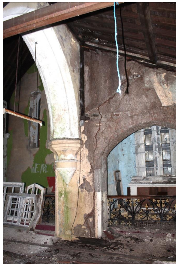
Plate 24: Severe moisture ingress at junction of wall separating southern aisle from southern side altar and south wall of nave with damaging vegetation exacerbating decay of plaster surface and masonry.
