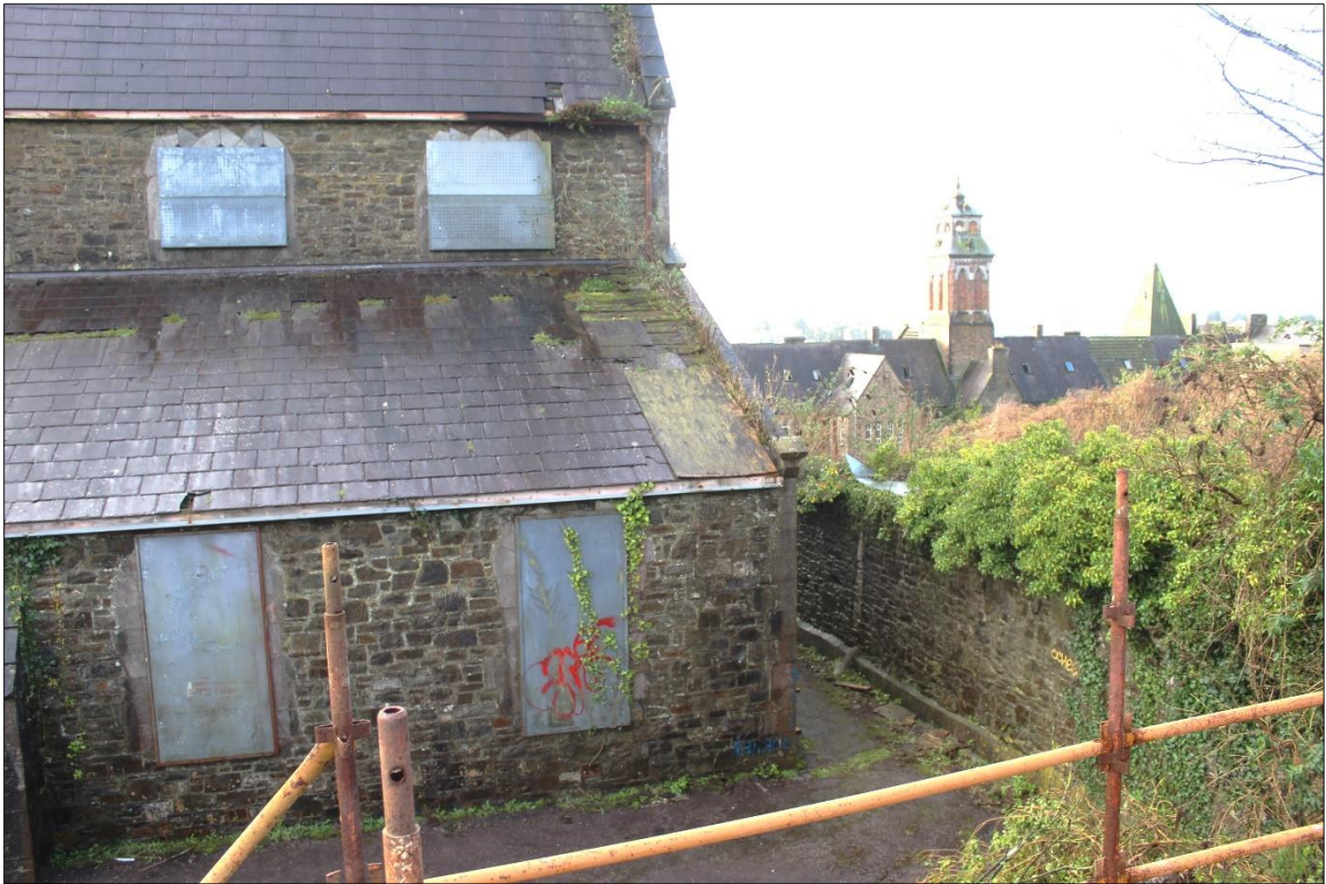
Plate 17: Area of missing slates at west end of northern aisle
