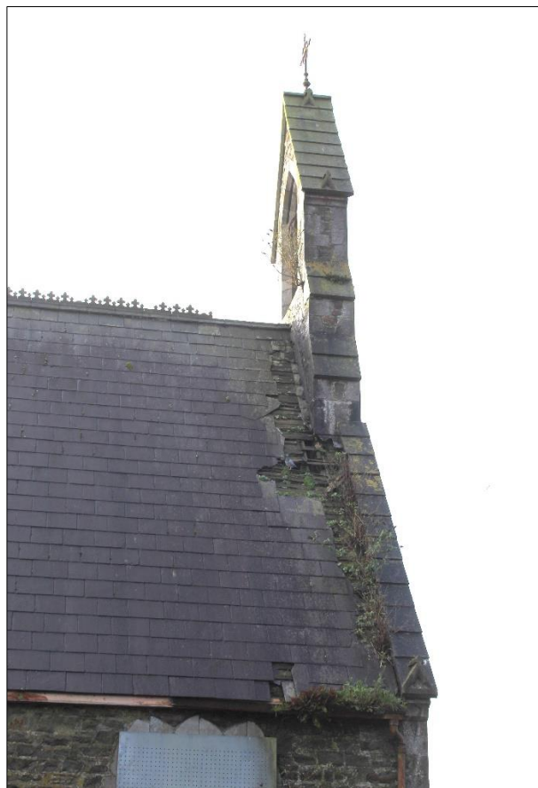
Plate 18: Area of missing slates at west end of main nave roof on northern elevation
