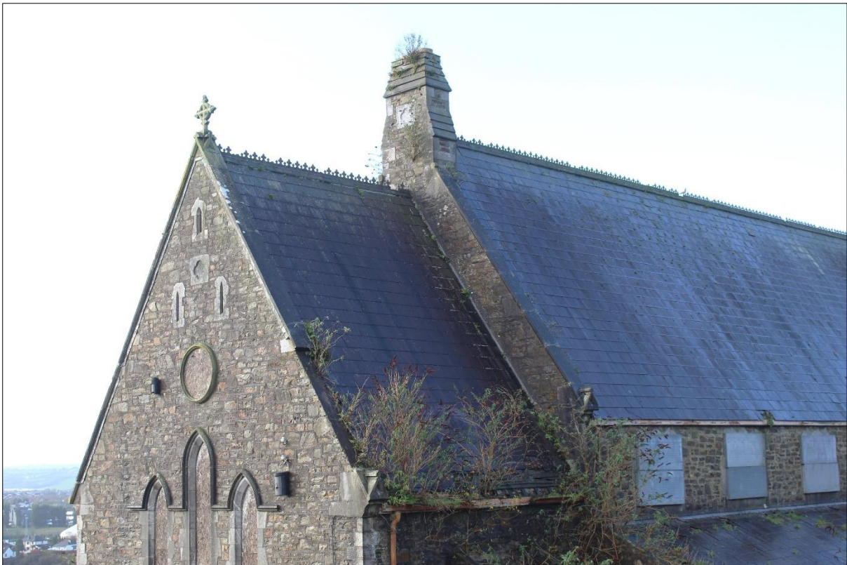
Plate 10: Detail of east gable masonry, chimney over chancel arch and damaging vegetation growth to exposed wall-tops on north elevation and lower portion of east gable wall of sanctuary
