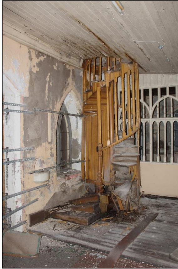
Plate 29: Badly-decayed timber spiral staircase to west balcony
