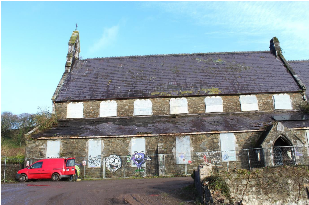
Plate 2: Southern elevation with large area of missing slates to western side of aisle roof
