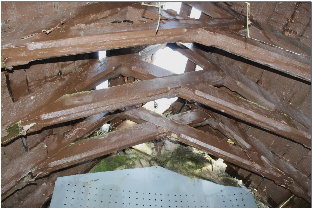
Plate 20: Detail of exposed underside to chamfered timber structure of damaged, roof to southern entrance porch.
